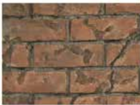
Cracked Red Fire Brick
